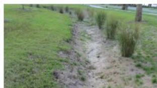
8 INLET EROSION (GRASS CHANNEL)
