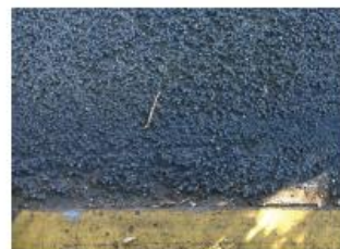
16 SMEARING (POOR) (COVERED WITH ASPHALT SEALER)
