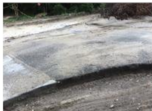
5 UNSTABLE DRAINAGE AREA & 13 SEDIMENT (POOR)
