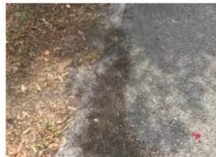
5 UNSTABLE DRAINAGE AREA & 14 DEBRIS (MARGINAL)
