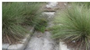
5 INLET STRUCTURE DEBRIS & SEDIMENT
