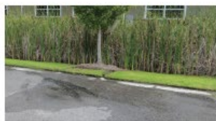
11 EXCESSIVE PONDING (CATTAILS & STAINING)
