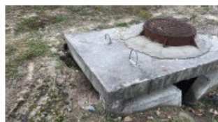
19 OUTLET STRUCTURE EROSION
