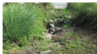
8 INLET EROSION (ROCK PLUNGE POOL)
