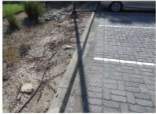
5 UNSTABLE DRAINAGE AREA
