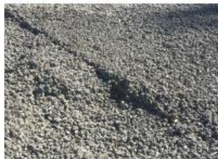
7 CRACKING & 15 RAVELING (POOR)
