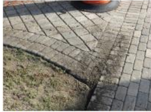
5 UNSTABLE DRAINAGE AREA
