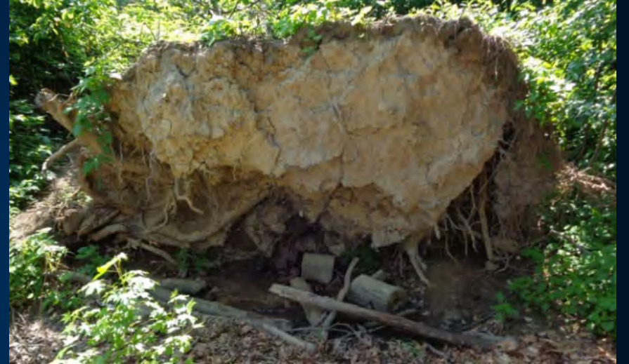
Uprooted tree in existing swale with signs of mottled soil around its roots and standing water
