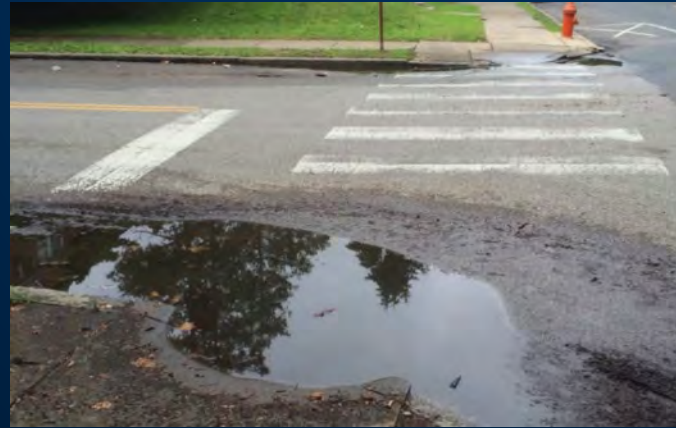
Ponding adjacent to curb ramps at the corner of Van Kirk and Charles Streets
