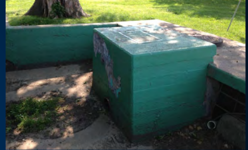
Outlet control structure located at low-point of hockey rink and basketball courts
