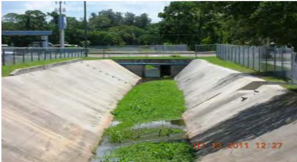
Figure 6: Ditch #5 in Pinellas County, Florida, is a manmade stormwater conveyance that discharges through a wetland into a navigable creek. It is already regulated as a point source. Under the Rule, it will be additionally regulated as a “water of the United States.” Fla. Stormwater Ass’n Comments 13
