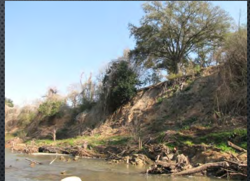
Eroding riverbank on Buffalo Bayou
